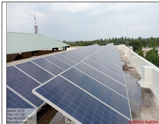
Solar Panel on Main Building
