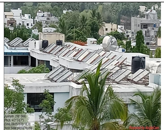
Solar Panel on Hostel
